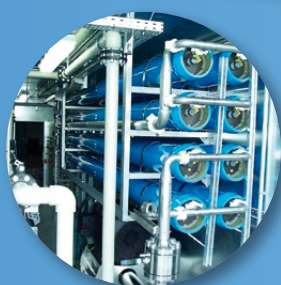
Container Unit, type SRO 300 m 3 /d, built in a 30 ft. insulated container incl. heating and ventilation for outdoor installation on a north sea platform.
